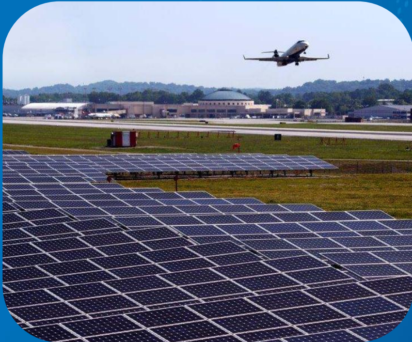
Chattanooga Airport 500 kW storage provides backup power to air traffic control.
